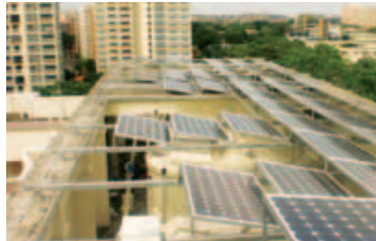
Figure 8.5 Solar PV system 3
