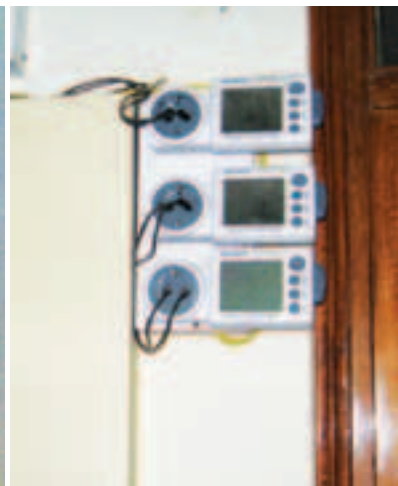
Figure 2.1c Energy loggers for monitoring electricity consumption of space-conditioning equipment
